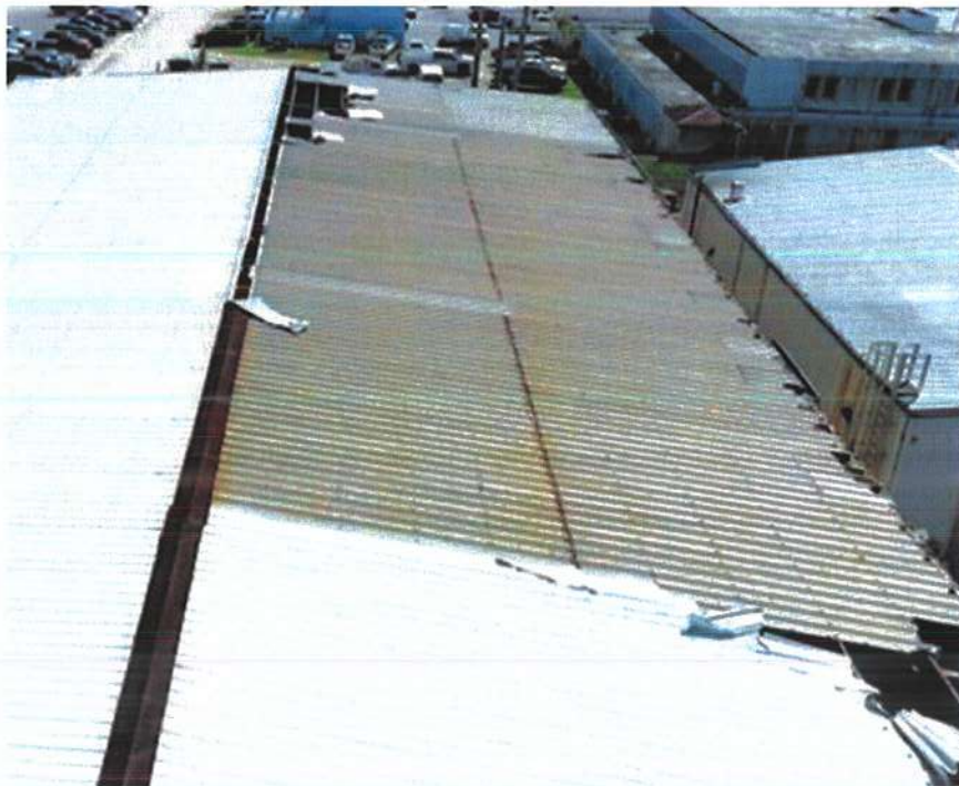
ITEMS 1 & 1A- DAMAGED ROOFING BACKSIDE
