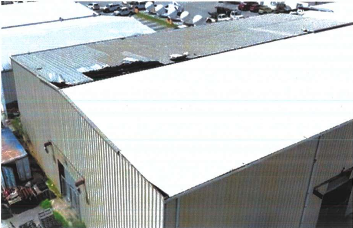
ITEM 6 – DAMAGED ROOF RIDGE
