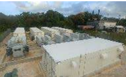
Talofofo BESS 16 MW Frequency Regulation
