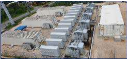
Hagåtña 24 MW Energy Storage Batteries
