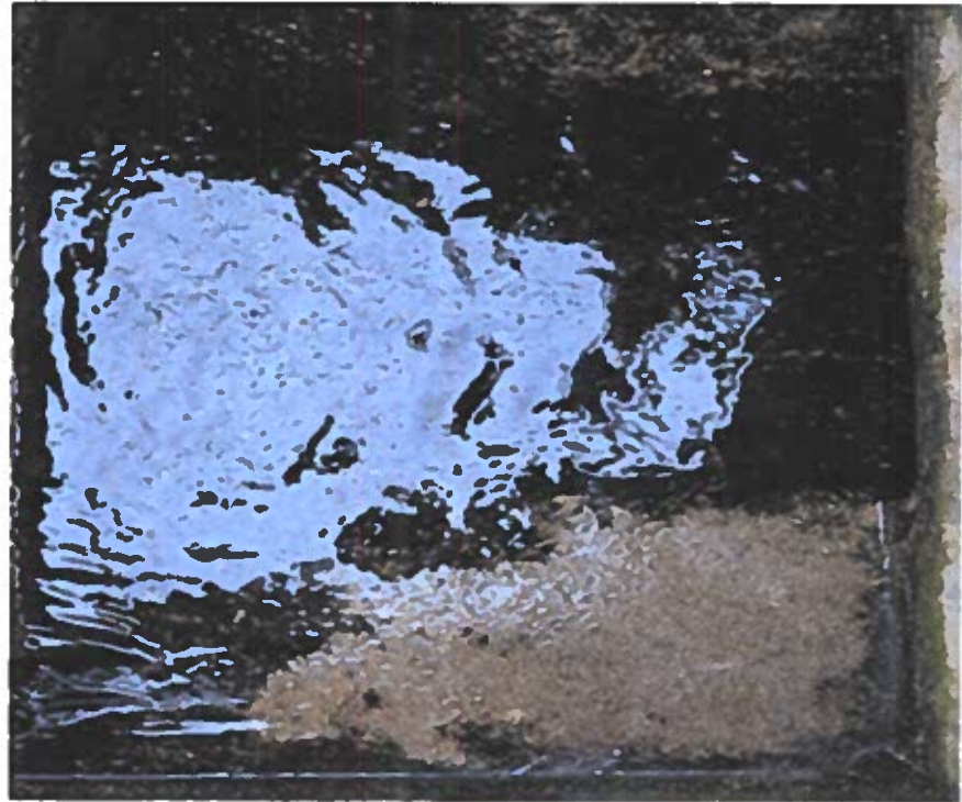
Temp. strainer (before reuse water pump)
