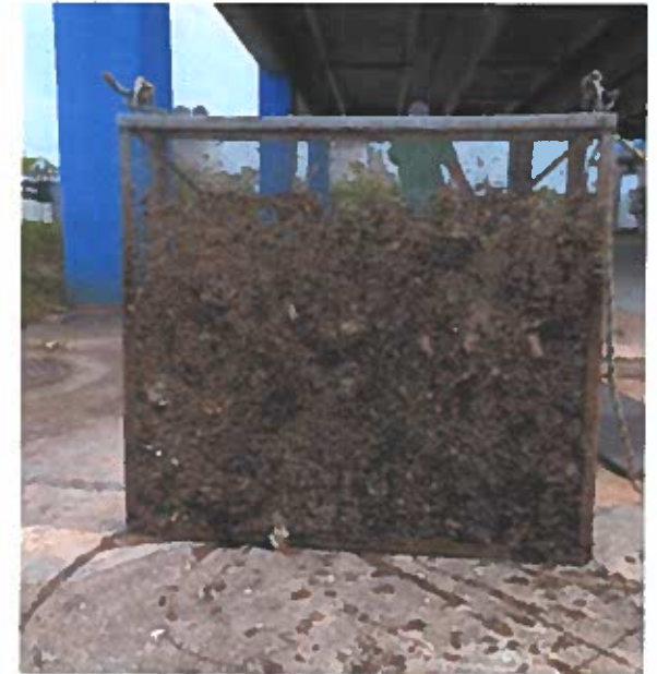
Large amount of debris - Nov. 07. 2025
